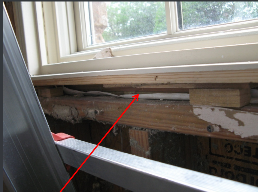
No sill flashing at window sill
