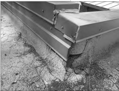
Degradation of the Building Envelope
