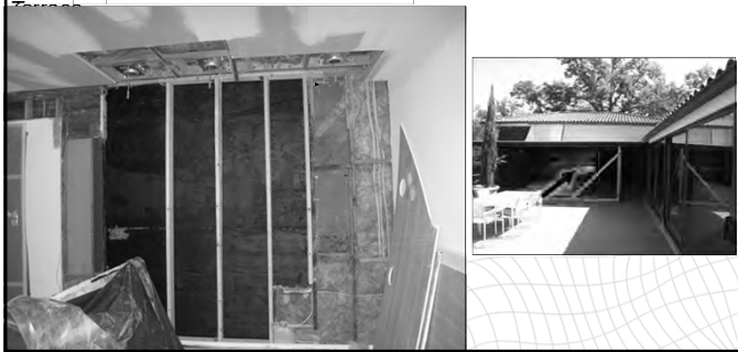
Moisture Distress and Replaced Framing Below
