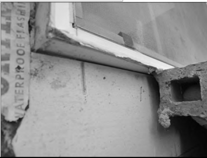
Improper Installation of Materials
