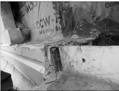
Improper Installation of Materials
